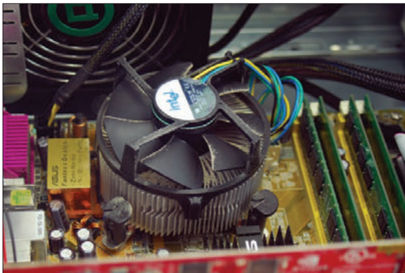
Figure 4-20 Dust in this cooler fan can cause the fan to fail and the processor to overheat
